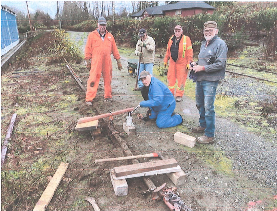
Salvage of track by the Machine Shop prior to excavation of bank by the Loci shed by Town contractors – this not only salvaged the trackage, but also saved the Town the cost of track removal.
